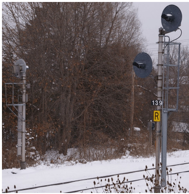
ABS signals located on separate masts on opposite sides of a single-track line.
