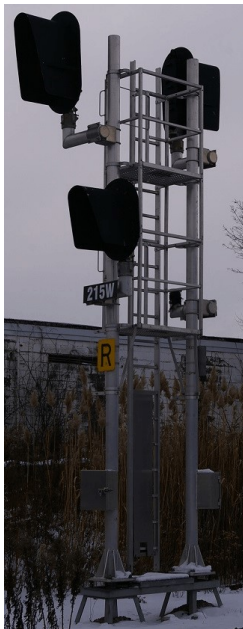
ABS signals mounted back-to-back. Upper staggered head (left) and single head mounted away from track.
