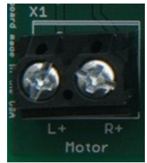
Figure 5: Motor Terminal Block
